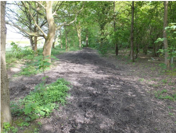
Muddy surface of BP1642 just East of Downslink – needs improvement for year-round commuter cycling
