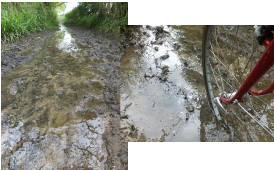
Current bridleway condition unsuitable for cycling
